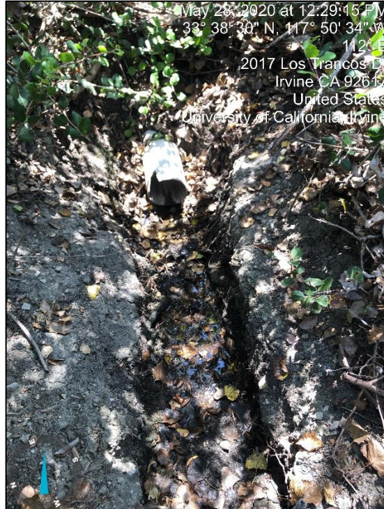
Existing storm drain inlet located on the downstream end of the drainage.
